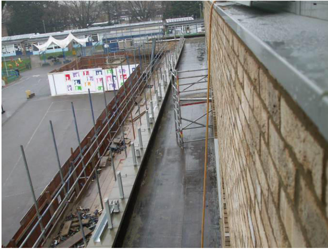
Photo 12 - Rear Balcony DHB viewed from a second floor window.
