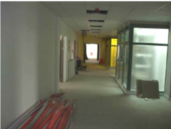
Photo 4 – 1 st floor corridor – part-painted
